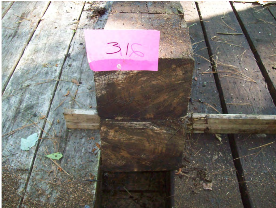
Figure 8 - Tie #31 red oak/creosote 7lbs (Koppers).
