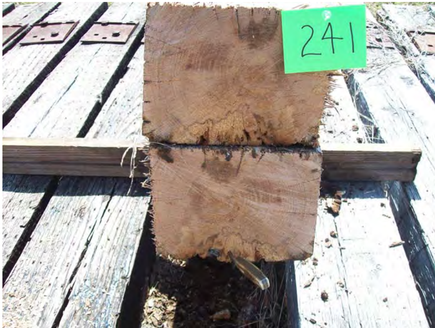
Figure 104 - Tie #241 untreated red oak with decay.
