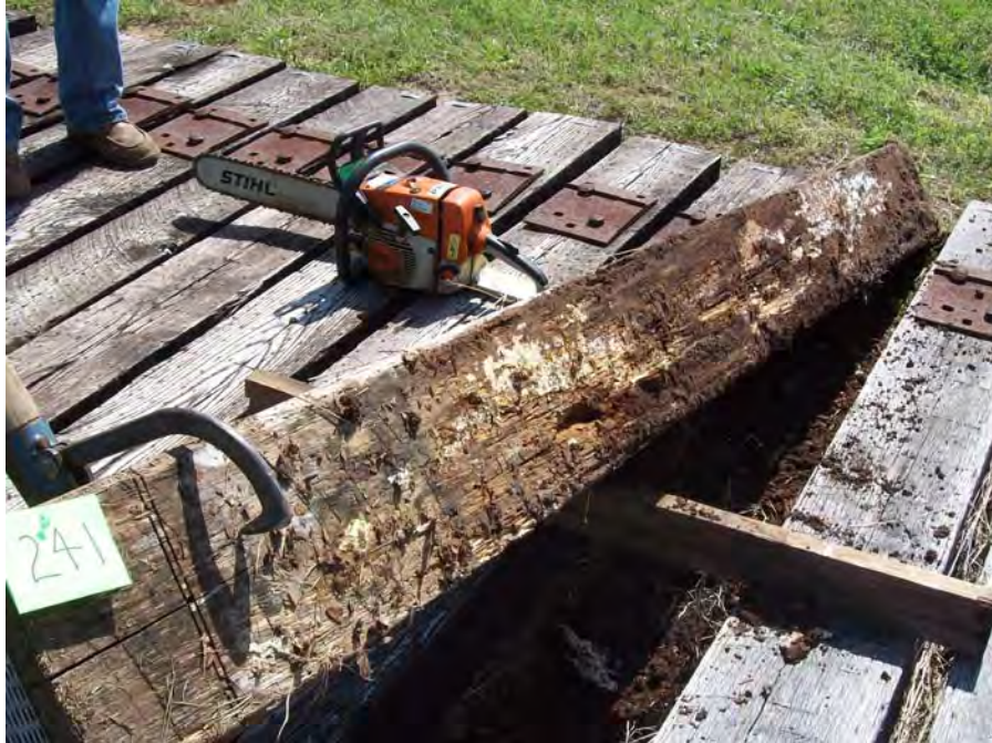
Figure 103 – Tie #241 untreated red oak with decay.
