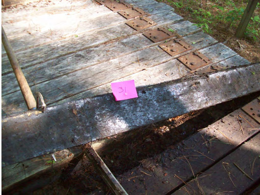
Figure 7 - Tie #31 red oak/creosote 7lbs (Koppers).
