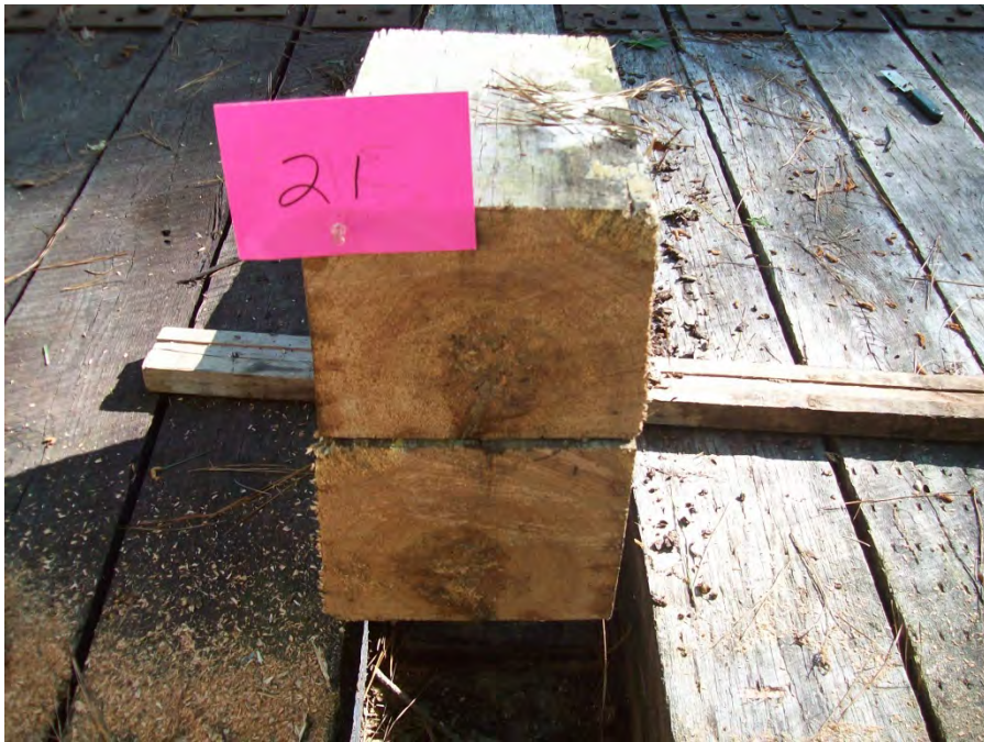
Figure 6 – Tie #21 untreated red oak with decay in multiple places.
