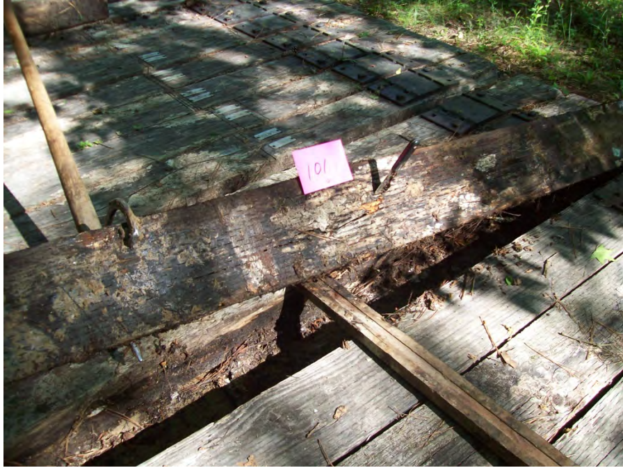
Figure 21 – Tie #101 untreated Douglas fir with decay.
