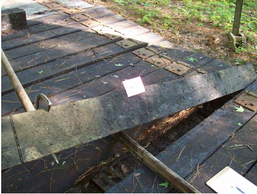
Figure 9 - Tie #41 white oak/borate/creosote 7lbs (Koppers).
