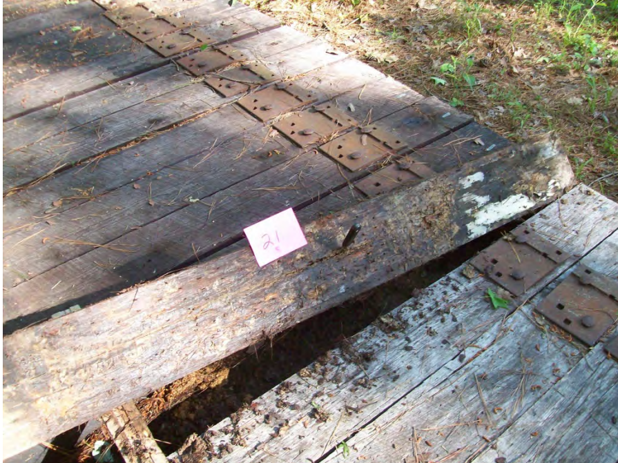
Figure 5 – Tie #21 untreated red oak with decay and termite damage.
