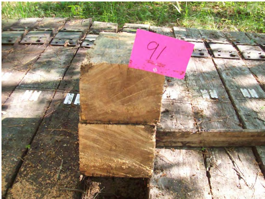
Figure 20 – Tie #91 untreated white oak with light decay visible.
