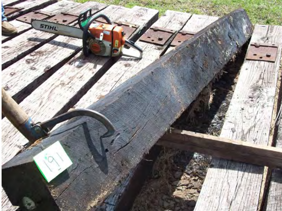
Figure 93 – Tie #191 white oak/creosote/6lbs (Koppers).
