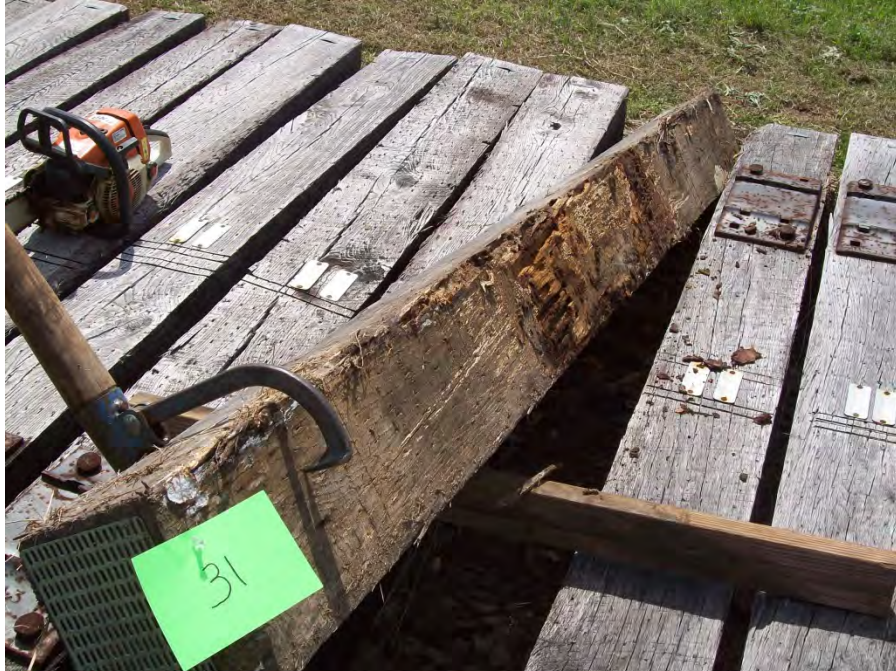
Figure 59 – Tie #31 untreated white oak with decay and beetle damage.
