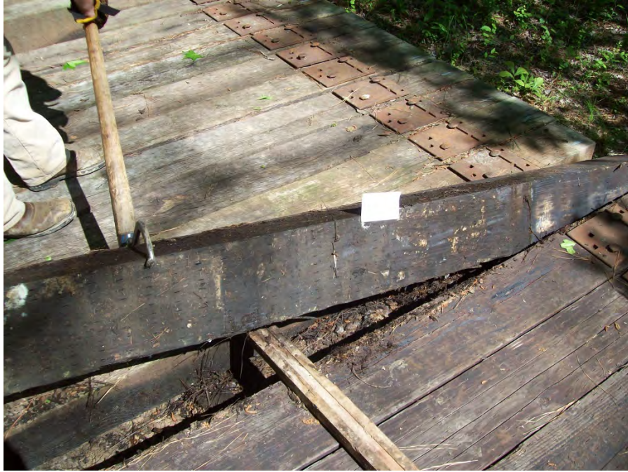
Figure 39 – Tie #181 Douglas fir/P2 creosote (Lonza).
