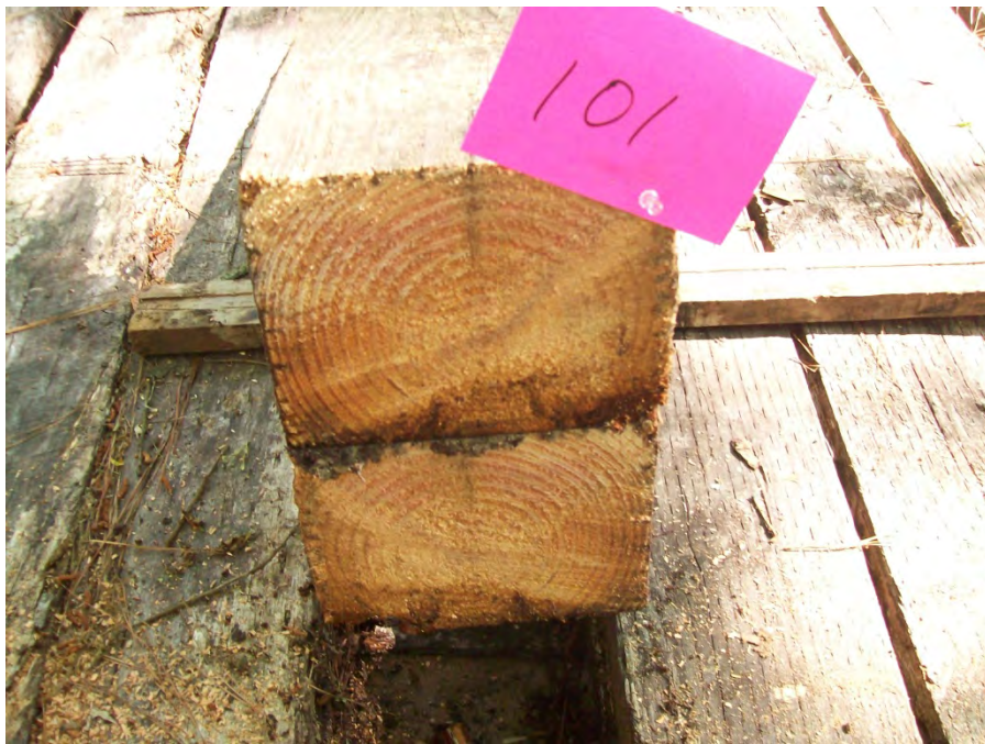
Figure 22 - Tie #101 untreated Douglas fir with decay.
